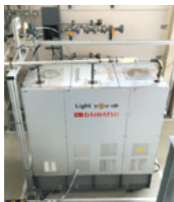
Biogas power generator
