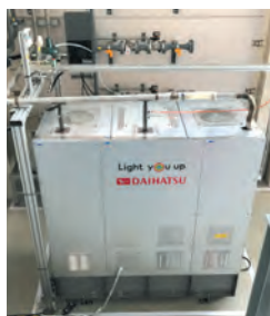
Biogas power generator
